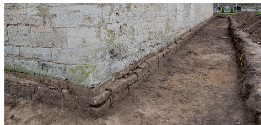
Fig. 4. View of the protruding foundation wall built of unhewn limestone on the southwestern side of the Konventhaus .
